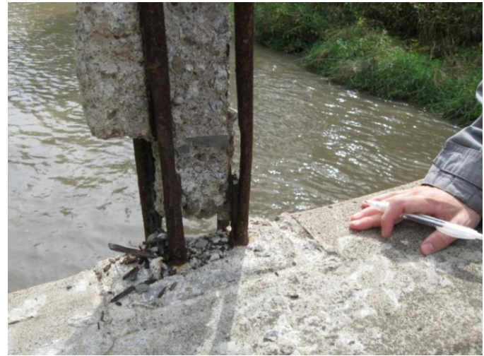
Figure 9. Vertical Spandrel Member showing Severe Spalling
