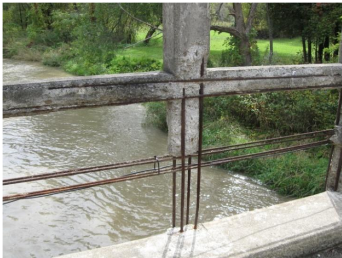
Figure 10. Vertical & Horizontal Spandrel Member showing Severe Spalling
