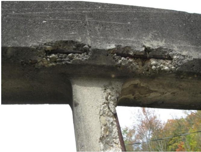
Figure 8. Truss Top Chord Showing Spalling
