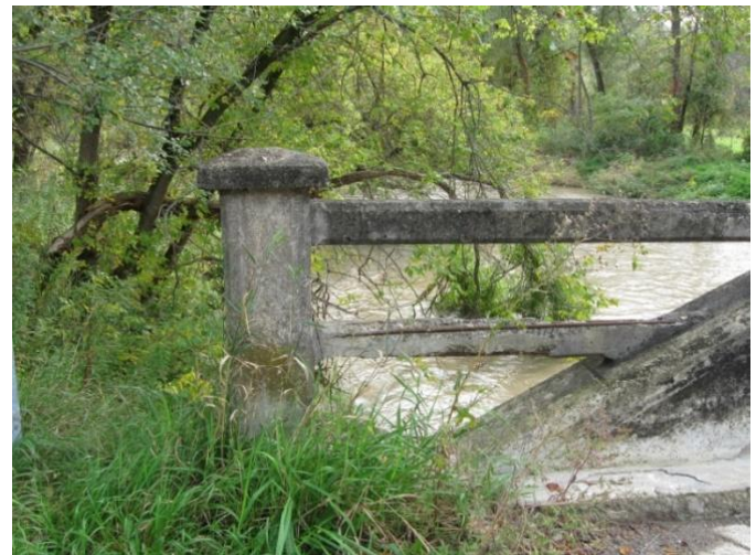
Figure 11. Handrail showing Delamination
