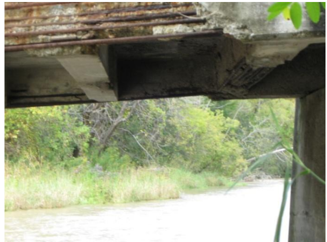
Figure 7. Cross Beams Showing Spalling
