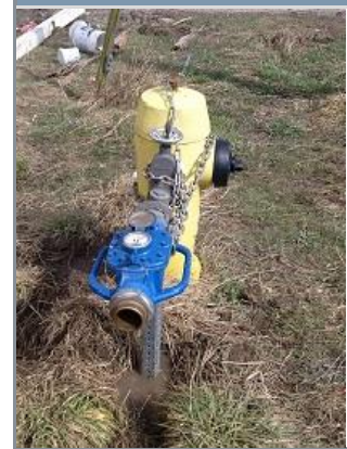
HYDRANT PREPARED FOR SAMPLING
